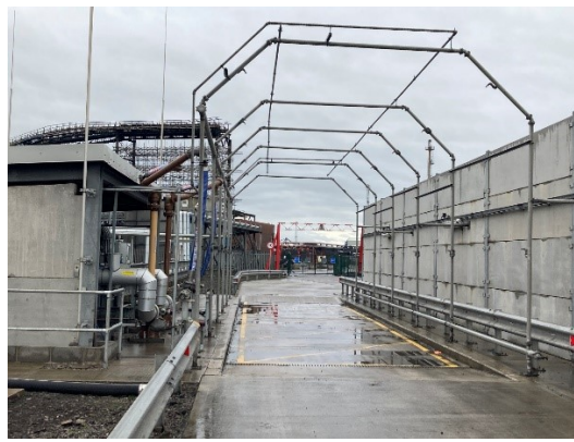
Figure 4: Benzole tanker loading area case study project photograph.
